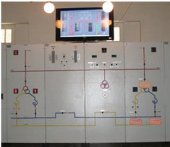
Fig. 1. High voltage substation control shield with additional monitor
